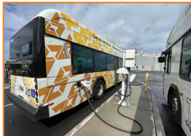
Photo above: E-bus plugged in at a charge station at the Kalihi Facility.
